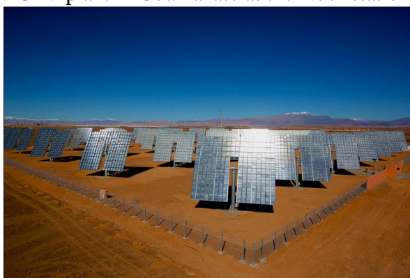
Fig. 9. CPV plant in Noor IV Ouarzazate
